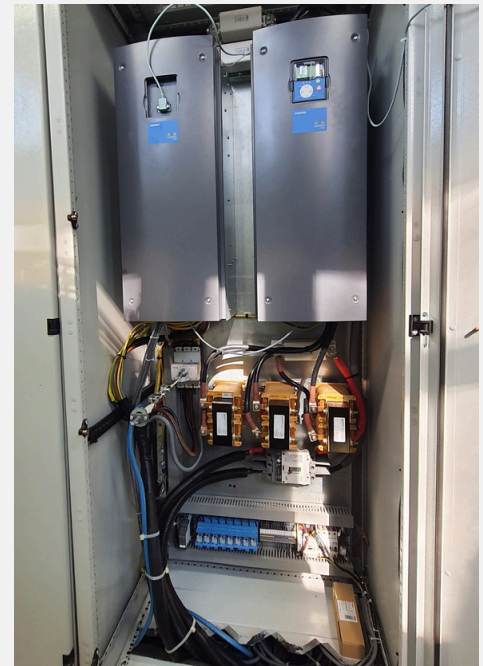
Photo: 75kW pump control system using VACON (Danfoss Drives) frequency inverters and Elhand's DC reactors
