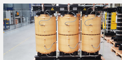
Photos: LOTOS Petrobaltic S.A/Elhand Transformatory
